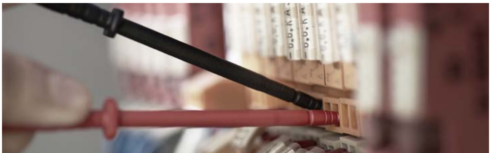
Measurements in fuse boxes and switch cabinets
